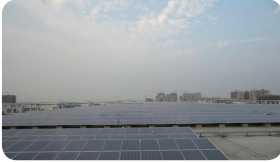
Huawei solar power station
